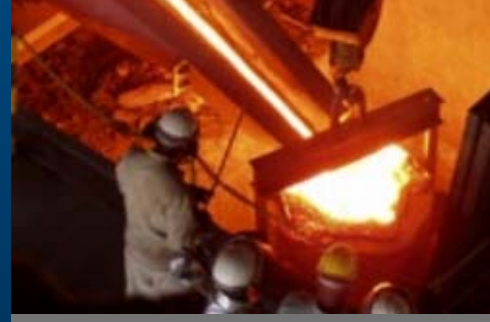
4MVA COPPER SMELTING PLANT
